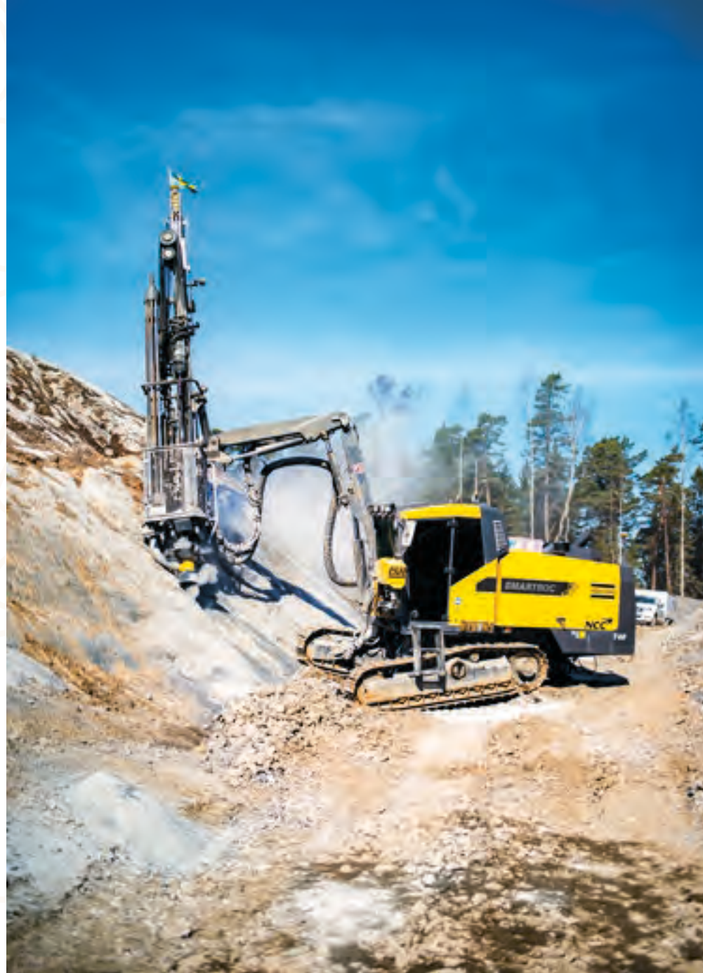
The explosives team (top left) | Meticulous coordination was needed to ensure safety during blasting and to handle the blasted rock efficiently.
