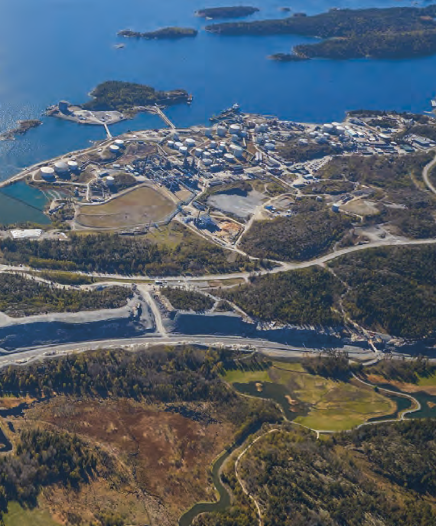
Stockholm Norvik Port May 2020 | The container terminal is ready for use. At the RoRo terminal the work to lay the paving stones is still in progress.
