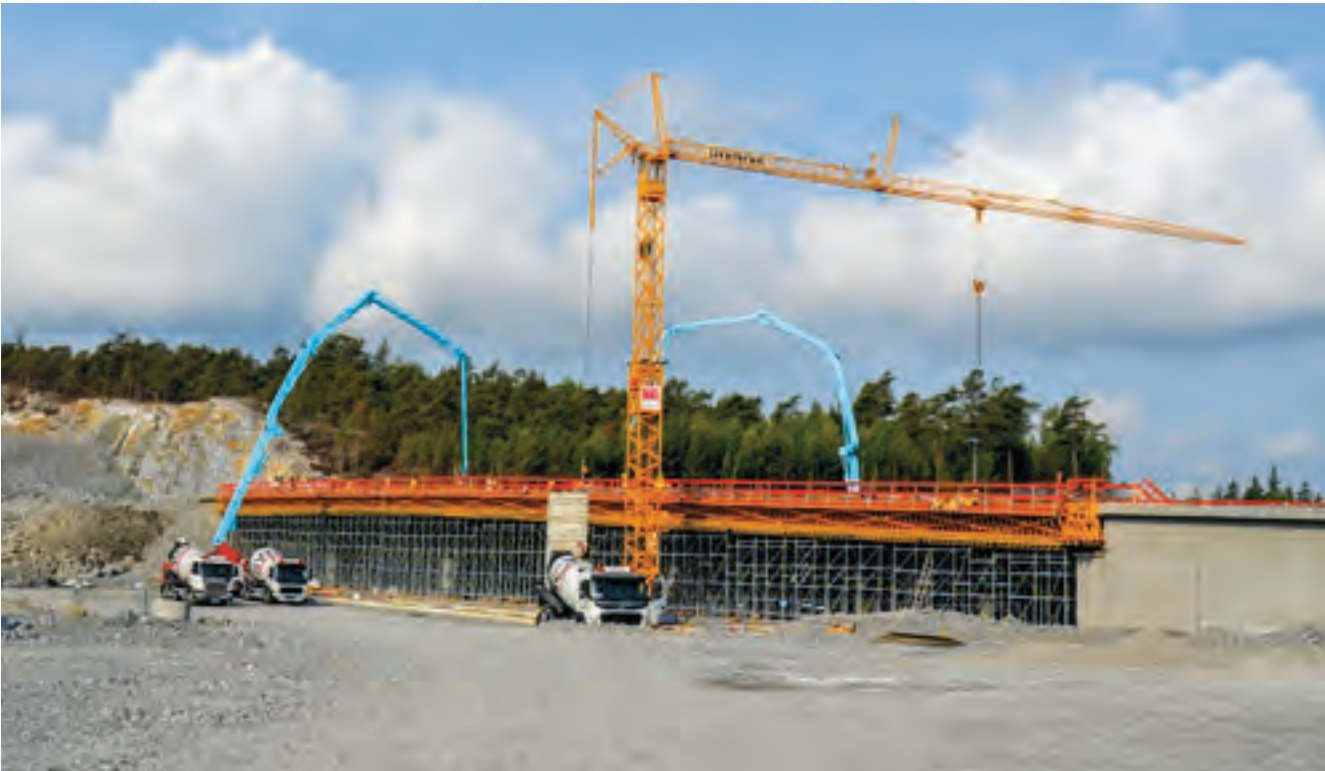
Access bridge (pages 120–121) | The bridge leading to the port separates the road and railway traffic. It also means there is no need to turn into, or cross, oncoming goods traffic. Traffic can flow unhindered. Four rows of pilings support the bridge erected in August 2018. One hundred metres long, five lanes wide, with a separate pedestrian and cycle overpass, the bridge needed two concrete pumping trucks and 2,200 m 3 of concrete on that single day of casting. When the concrete was in place it was watered to prevent the risk of fissures forming if it set too quickly. In total the construction of the bridge required around 3,800 m 3 of concrete.
