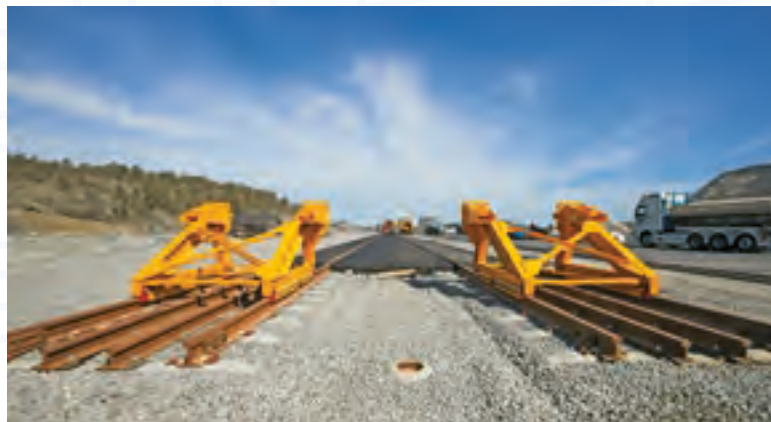
Station Norvik (pages 102–103) | The Norvikbanan railway ends in two 360 metre-long loading and unloading tracks in the container yard. Having the track level the same as the road surface makes it easy for trucks to load and unload goods. No heavy vehicles cross the tracks, so tarmac is enough to support the rails here.
